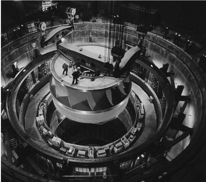
Figure 8.5 A Francis turbine runner, rated at nearly 1 million hp (750 MW), being installed at the Grand Coulee Dam, United States. (Image provided by the U.S. Bureau of Reclamation is in the public domain, http://en.wikipedia.org/wiki/Water_turbine )
