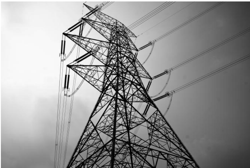
Figure 13.18 High voltage transmission lines.
