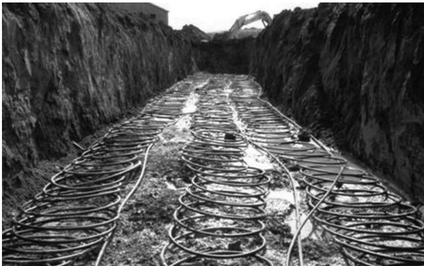
Figure 6.11 A horizontal closed loop field is composed of pipes that run horizontally in the ground below the frost line—photo shows a “slinky” (overlapping coils) arrangement before it has been covered by dirt. The slinky style layout is a more space-efficient version of a horizontal ground loop than straight piping. (Image by Marktj released to the public domain; http://en.wikipedia.org/wiki/Geothermal_heat_pump )
